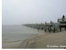
US Highway 90 in Mississippi, after Hurricane Katrina
