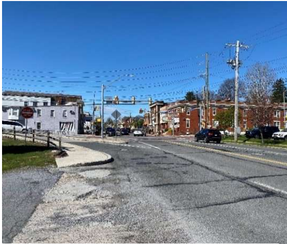
Inconsistent shoulder widths
