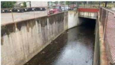
Photo 1: Looking towards Lafayette Street, several outfalls can be seen partially submerged in low flow conditions.
